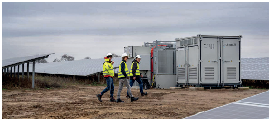
Sungrow's inverters SG3125HV-20 plus MV Skid on site (credit: BELECTRIC)
